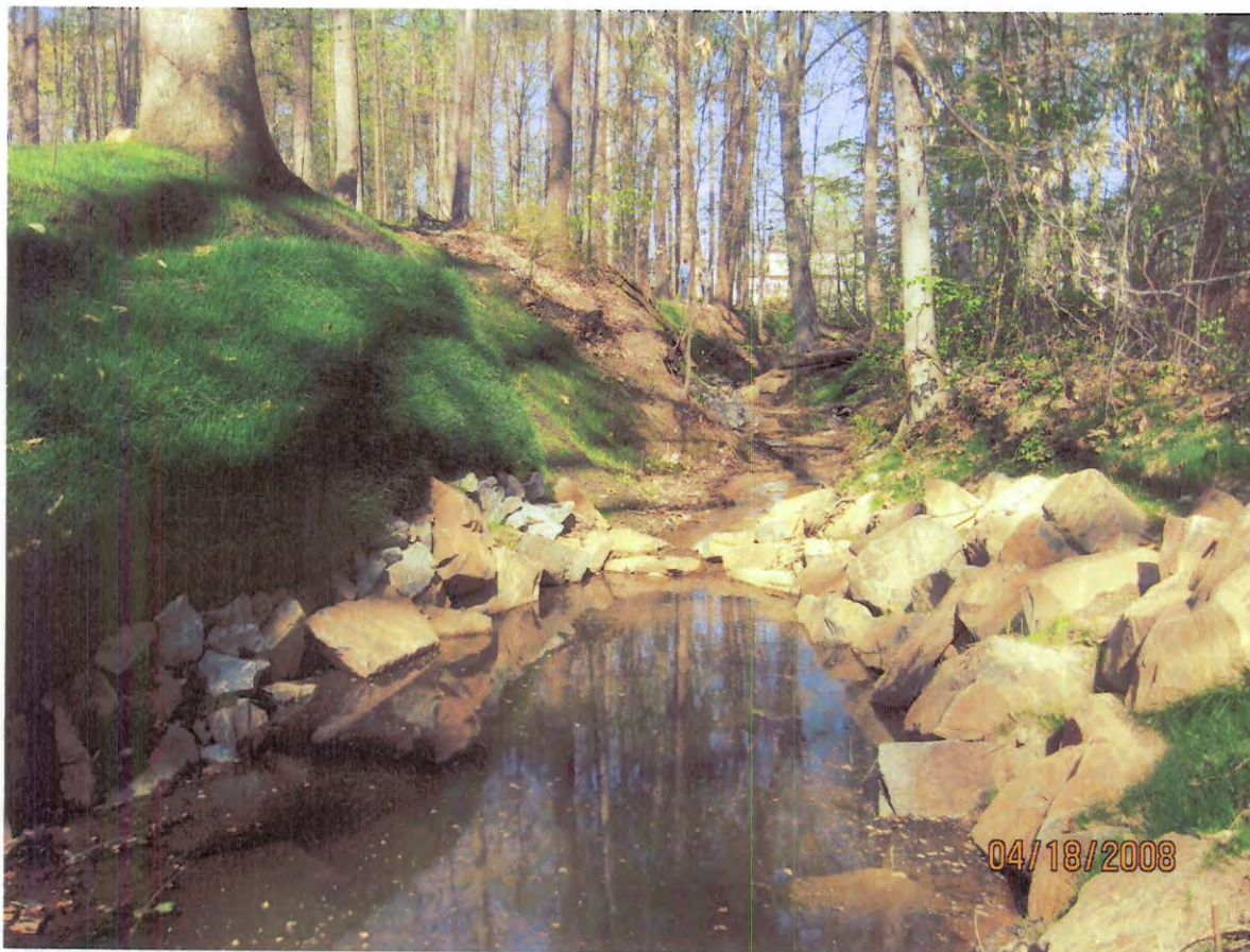
AFTER - left bank filtrex stabilization and right bank rock stabilization (below weir #2).
