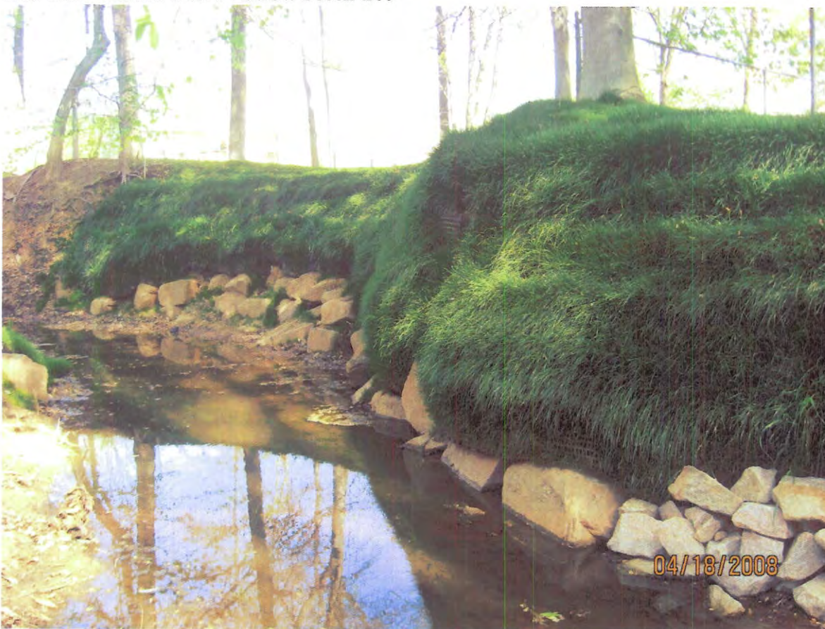
After- above weir #4 create large terrace sill by stone toe, back fill and filter fabric applications.
