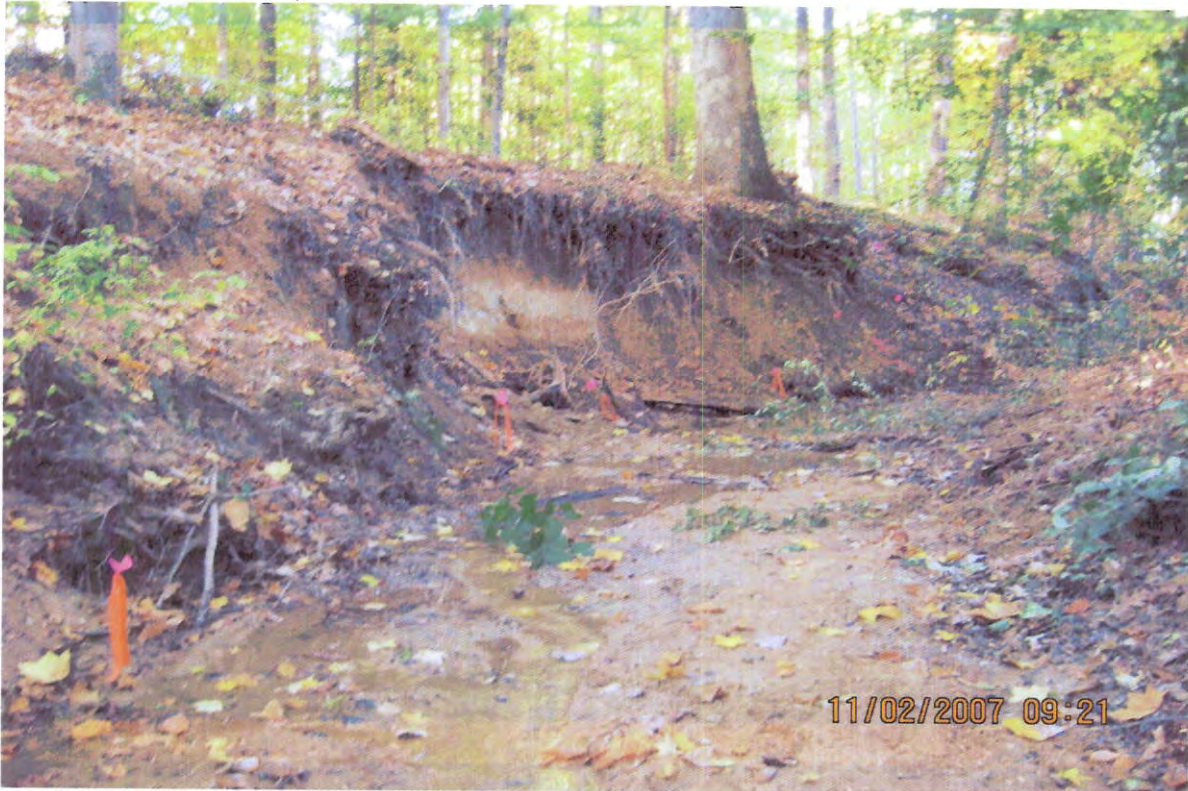
BEFORE – (Photo Zone 2) Future location of #2, rock weir and left bank stabilization.
