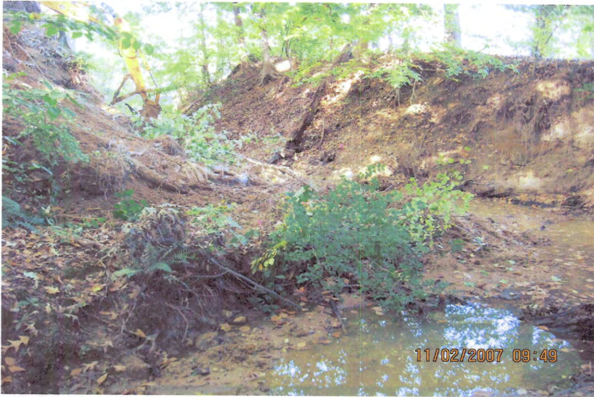
BEFORE - Location of "slope failure area" across right bank created sill and stabilization area.
