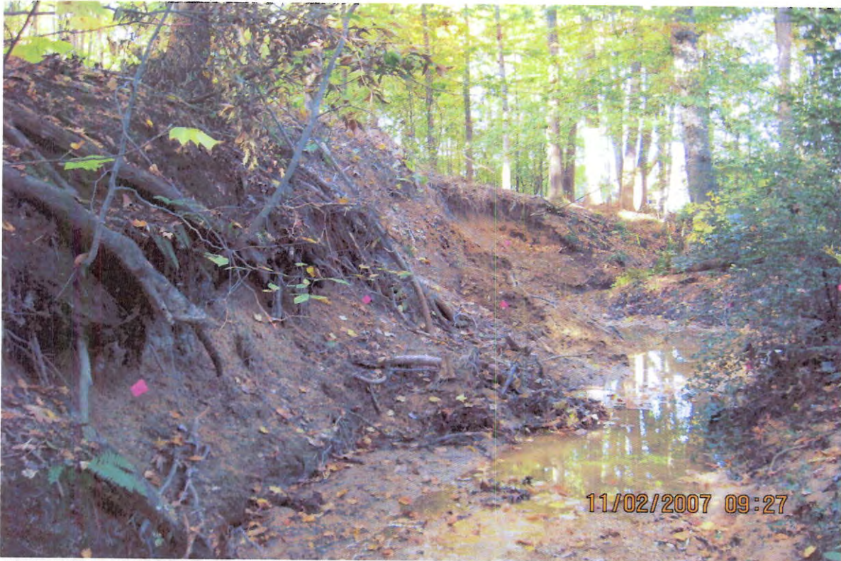
BEFORE – Left and bank needs stone toe filter sock and compost tea bank stabilization.
