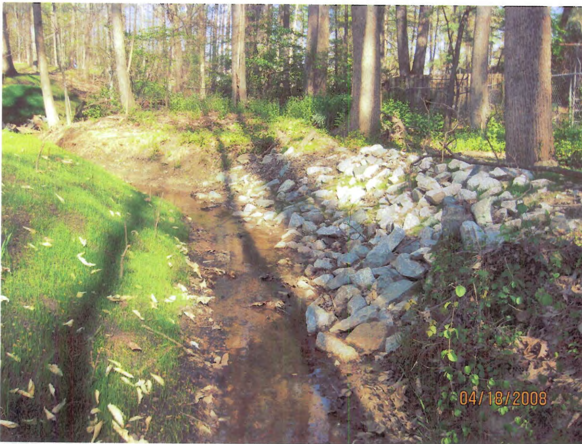
AFTER - Location #1, cut and fill of banks and stone and mulch bank treatment..
