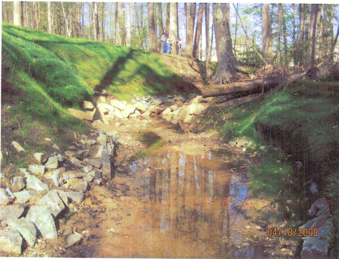
AFTER – Left and right bank stabilization with stone toe, filter sock and compost tea.
