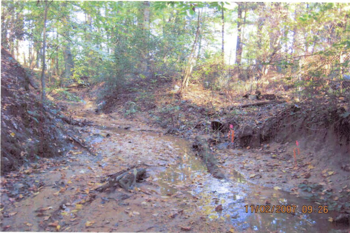
BEFORE – Right bank needs stone toe and bank stabilization.
