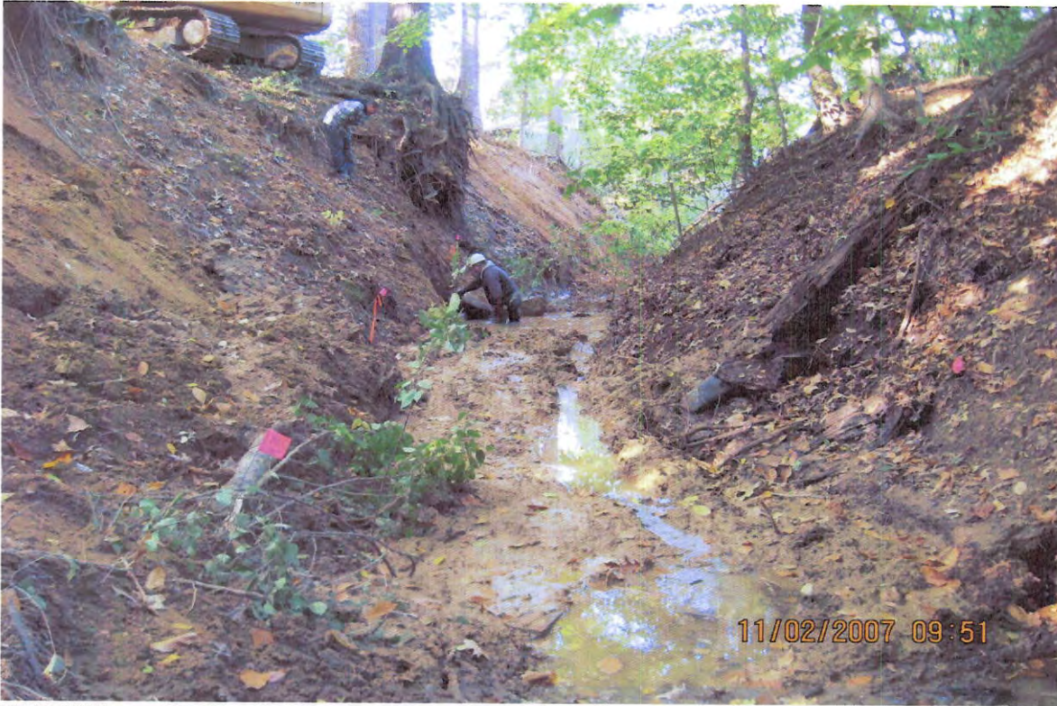
BEFORE –need stone toe treatment , grade bank and stream bank to be covered with compost tea.
