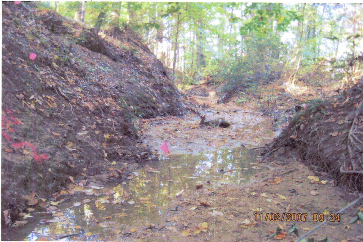
BEFORE – (Photo Zone 2) left bank stabilization and right bank stabilization (below weir #2).
