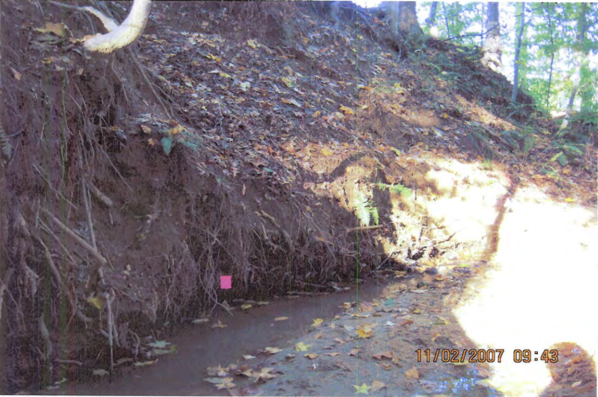
BEFORE - Need to create a stone toe and cut slope to terrace to support filterxx bank stabilization.
