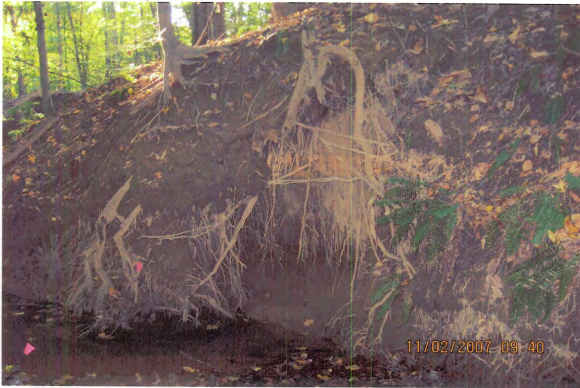
BEFORE – Need to stabilize bank with toe stone, filtrex sox and backfill.
